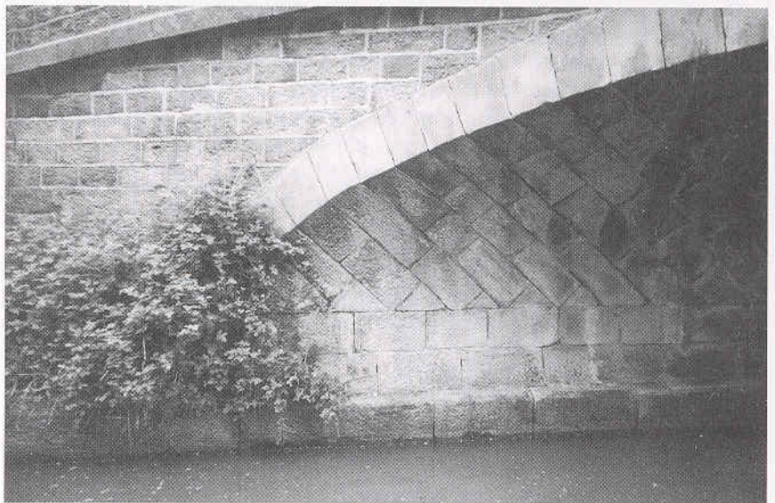
Two views of Bridge 26, where Sugar Lane crosses the Macclesfield Canal. The first stones here were cut at an extreme angle - impossible to judge beforehand, without the calculations described.
